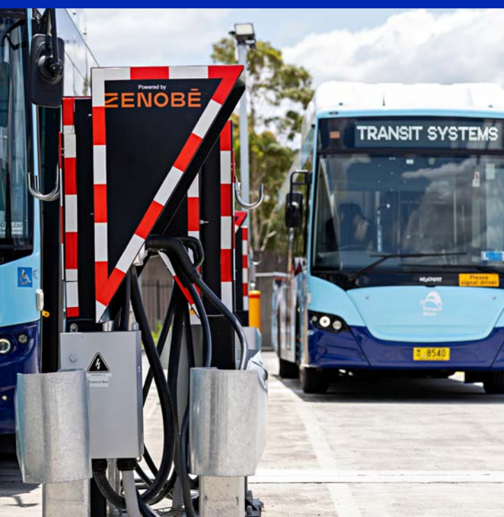
Zenobē-powered electric bus depot in Sydney, Australia.
